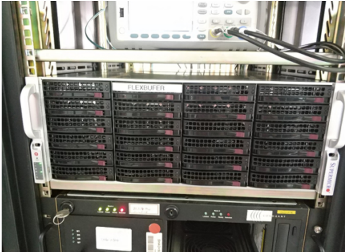
Figure 5.12: New FlexBuff hardware system at Tianma station.
