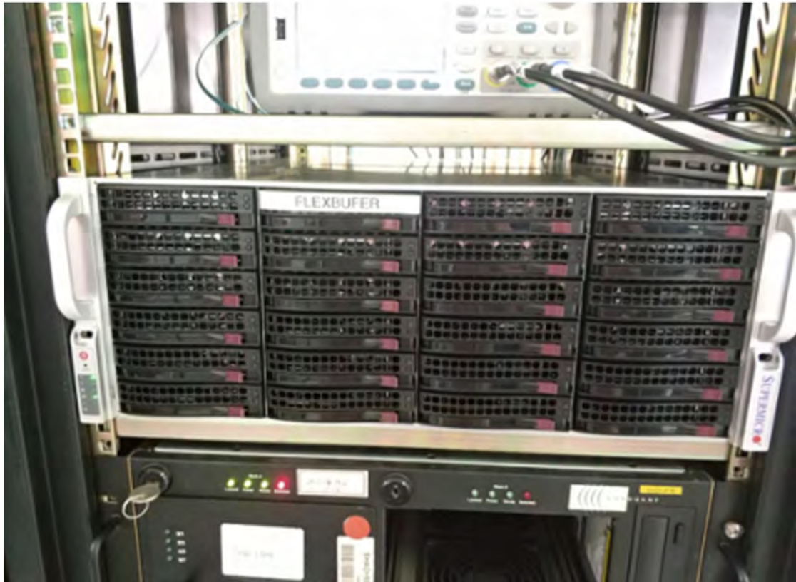
Figure 5.12: New FlexBuff hardware system at Tianma station.
