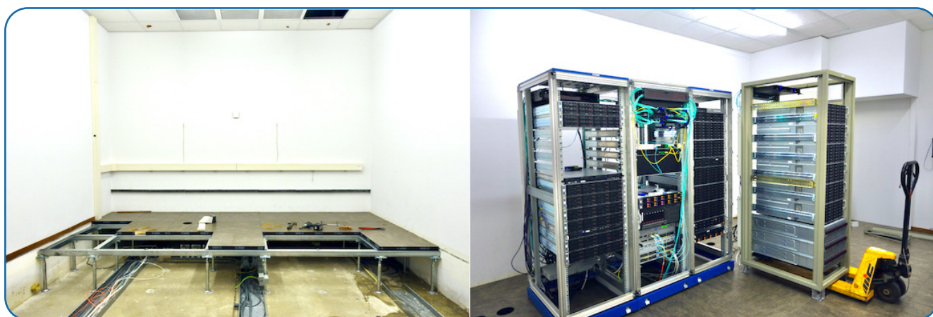
Figure 2: Left - The reinforced raised floor in progress of being installed. Right - A rack with several FlexBuff storage systems and software correlator microblade server chassis being put in its new position after the floor upgrade. The cabinet with the cyan fibers (2nd from the left) was offline for only two brief periods; it was relocated and reconnected with the highest priority because it contains the core switches connected to the 100 Gbps external link and servers running services such as Mattermost, ntp, ldap, databases and some webservices. Credit: Paul Boven.
