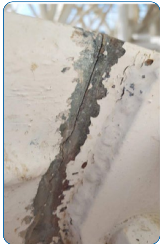
Fig. 1: Crack after the coating removal.
