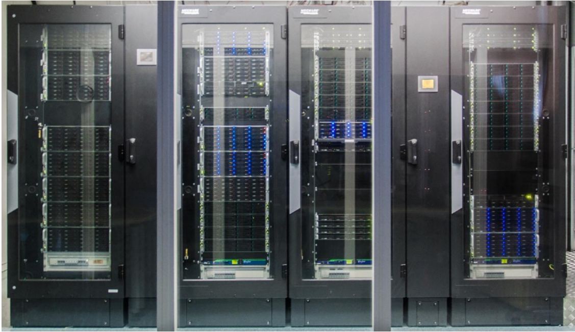
Figure 18: New computer cluster, January 2016 (photo H. Rottmann)
