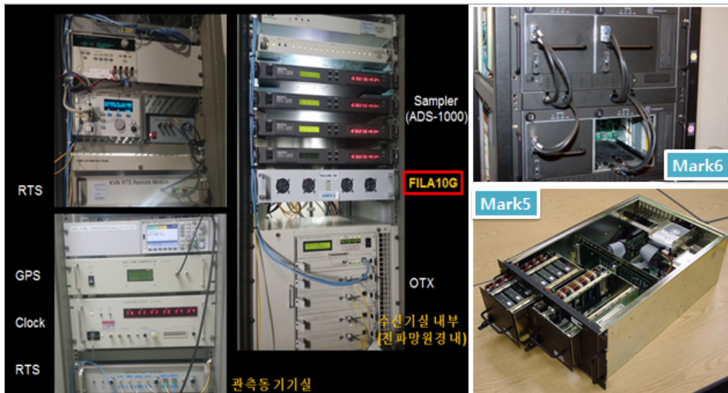
Figure 32: KVN data acquisition system with newly installed FILA10G and Mark6 systems
