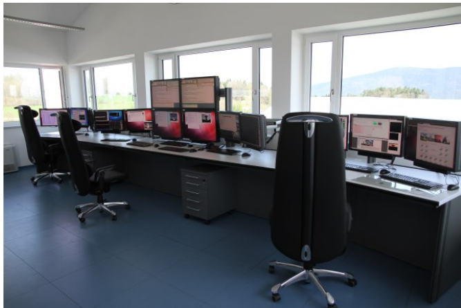
Figure 33: The new control room and data center in the Twin operations building.
