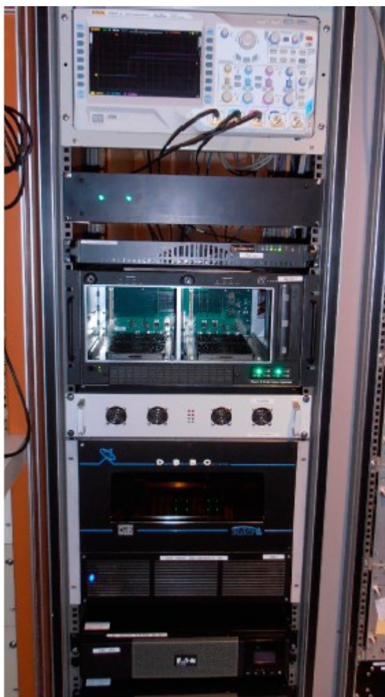
Figure 38: The new VLBI rack at Metsähovi.
