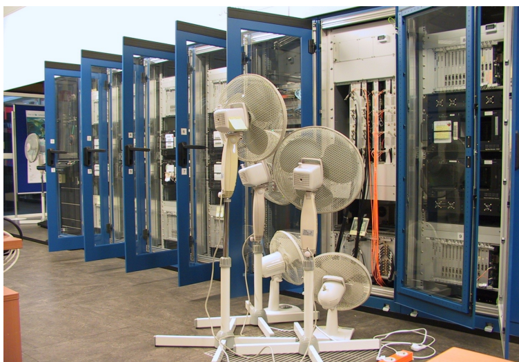
Figure 1: first e-VLBI test involving Badary during a cooling machine failure
