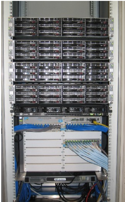
Figure 1: the SFXC cluster, consisting of four Transtec Calleo 642 servers. Each server contains four nodes, each node is equipped with two quadcore Intel Xeon 2.26 GHz E5520, giving a total of 128 cpu cores.
