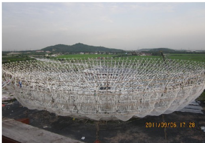
Figure 1: Shanghai 65-Meter Radio Telescope. (top): The mount of the telescope has been completed. (bottom): The assembly of the primary reflector structure has been finished on the ground and will be installed on the alidade of the telescope late this year or early next year.
