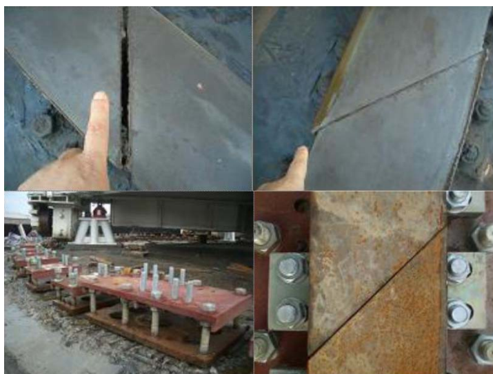
Upper panels: antenna track gap and offset. Bottom panels: repairing track in 2006.
