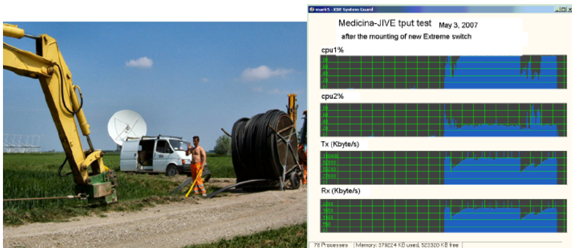
Fig. 6.4: Laying the fiber optic cable at Medicina and Test results Medicina-JIVE link
